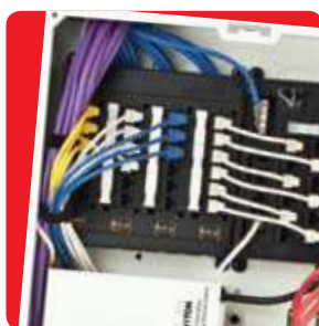
HOME WIRING & NETWORKING
