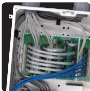
HOME WIRING & NETWORKING
